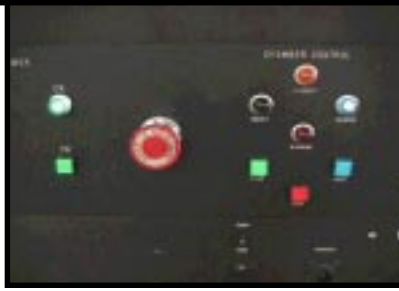
Chamber control panel.
